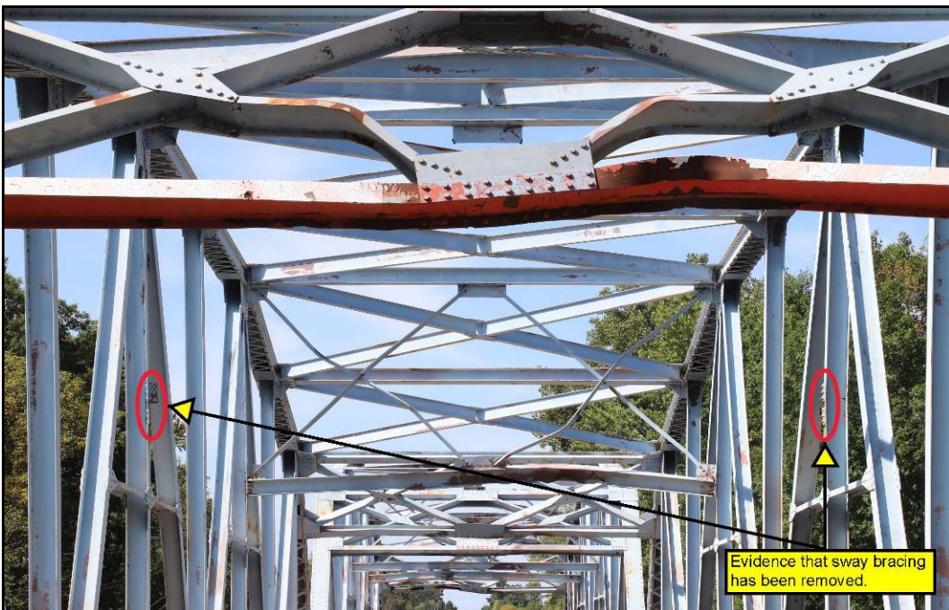
Figure 7: Note the loss of a complete sway bracing component in the easternmost span, as well as evidence of many significant hits to both portal and sway bracing elements.
