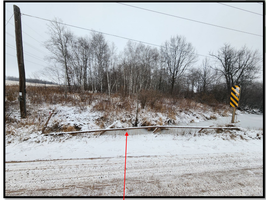
Damaged metal bridge rail
