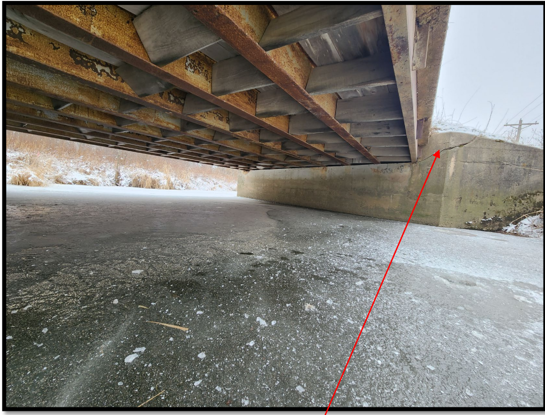
Cracks in abutments
