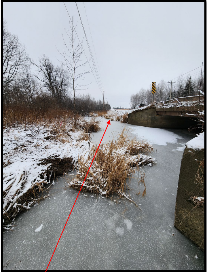
Existing Channel Flow, cutting into the roadway
